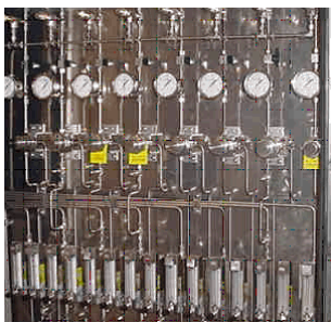
PurgeMaster 10A6100 in liquid sampling panel
